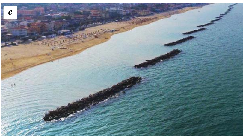
Fig. 2. Examples of coastal protection using natural stone: a – stone sloping revetments, Oregon (the USA); b – stone sloping revetments, Cyprus; c – breakwaters on the Italian Adriatic coast
