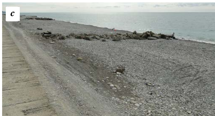
Fig. 4. Use of natural stone in Russian hydrotechnical construction: a – rubble-mound revetment at the right bank of the Nechespsukho River in the village of Novomikhailovsky (the Krasnodar Region); b – a rubble-mound groin with traverses in the village of Nebug (the Krasnodar Region); c – partly ruined rubble-mound groins at the Tuapse – Sochi section
